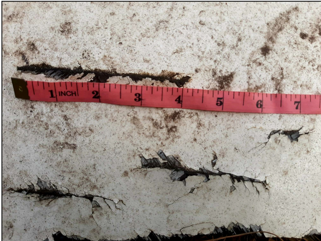
Figure 27: Close up of puncture damage white side up to 4" long.
