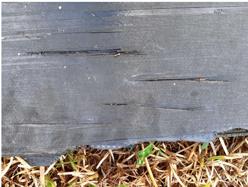
Figure 28: Close up of puncture damage black side (photo mirrored).
