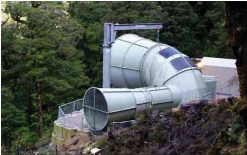
Figure 8.5: The surface back-up fan
