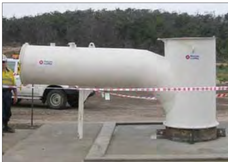
Figure 33.6: Inertisation connection facilities
